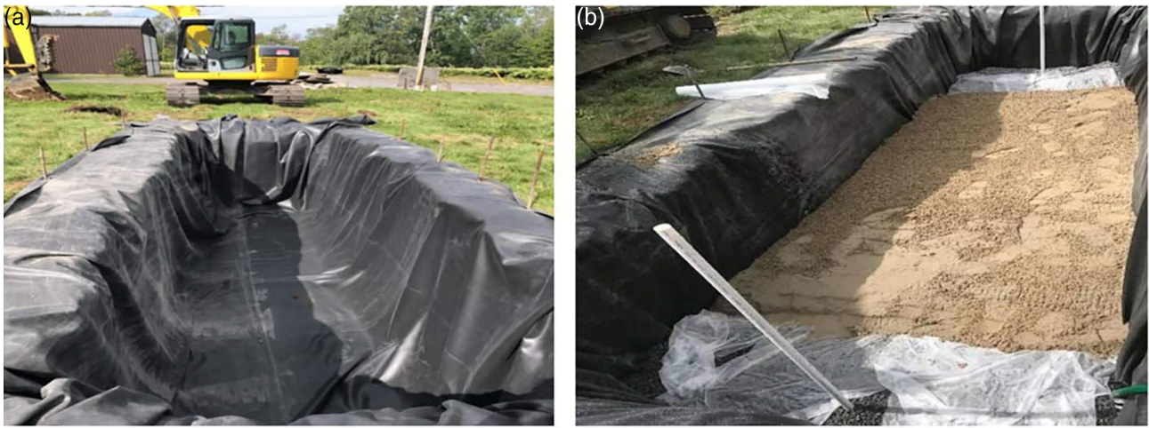
Figure 2. (a) Pilot-scale system test pit; (a) excavated pit was 6 feet deep by 6 feet wide by 20 feet long, lined with an EPDM pond liner, and (b) pit with packed sand before HRX well installation with 2-foot long gravel compartments at each end.
